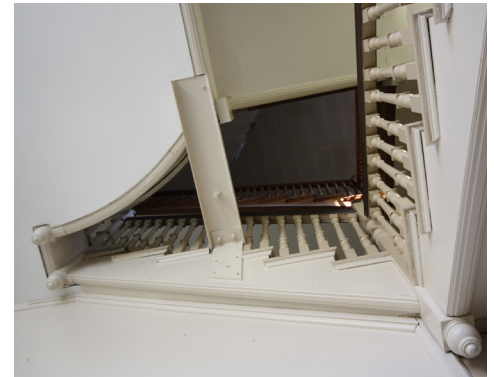
ATTIC/STAIRS IN NEED OF REPAIR
