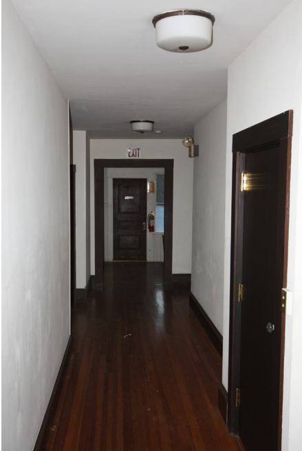
Interior partitions are not ideally suited for office suites. Re-planning of interior layout recommended.
